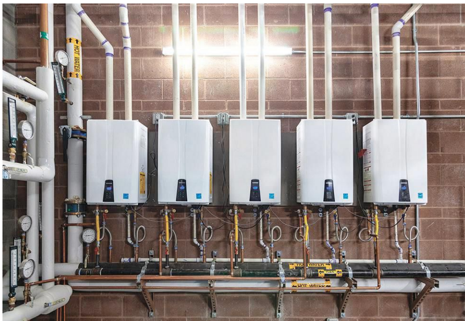
While the arena's water-to-water heat-recovery equipment supplies preheated water for the building's domestic hot water, the superheater only brings water up to a certain temperature, so designers specified a Navien NPE-240S tankless water-heater system to finish the task.
