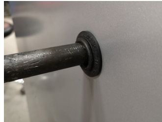
Figure 27. Furnace Gas Pipe Connections (Note Rubber Grommet)
